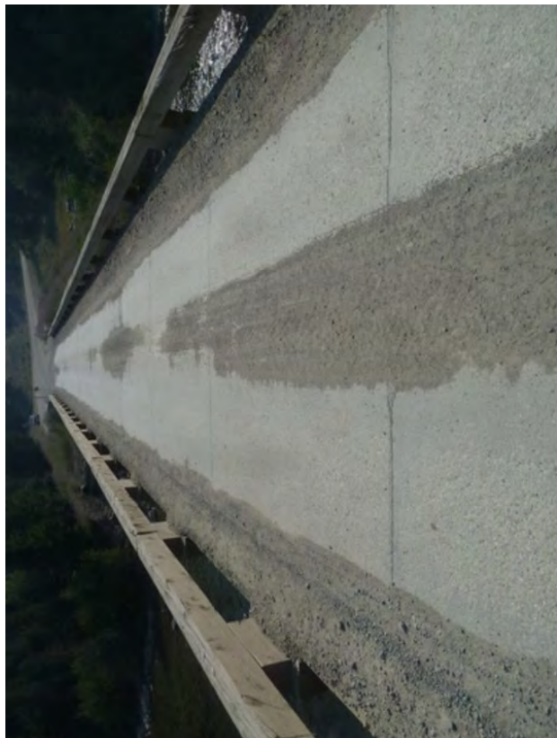
Figure 9: General deck condition - Note debris accumulation along deck edge and centre of deck - possible cause of noticeable wear.
