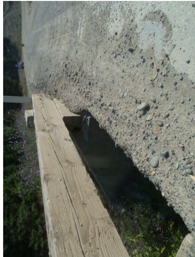
Figure 15: Failed curb riser at right end downstream.
