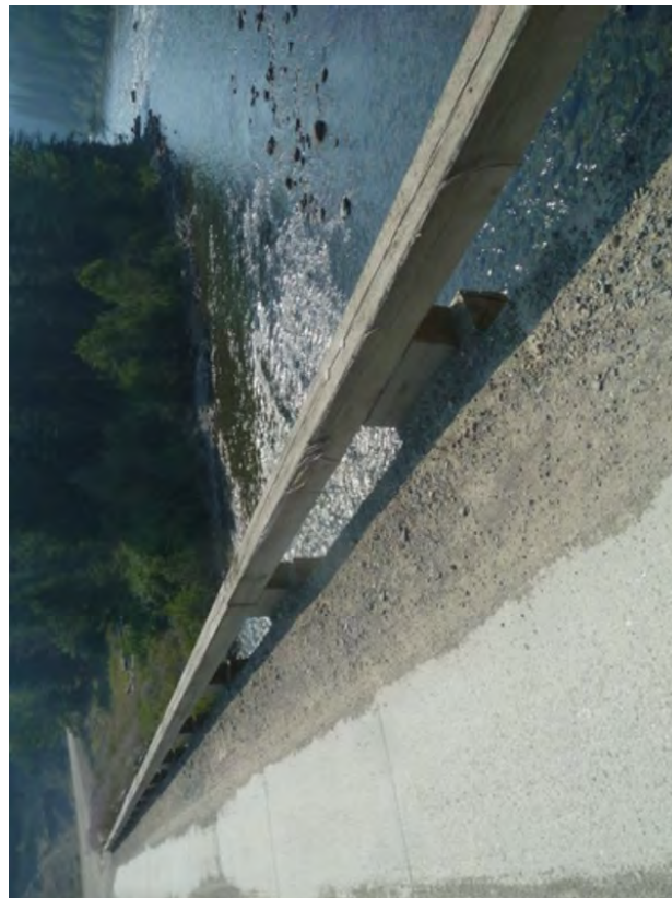
Figure 11: Typical condition of upstream curb.
