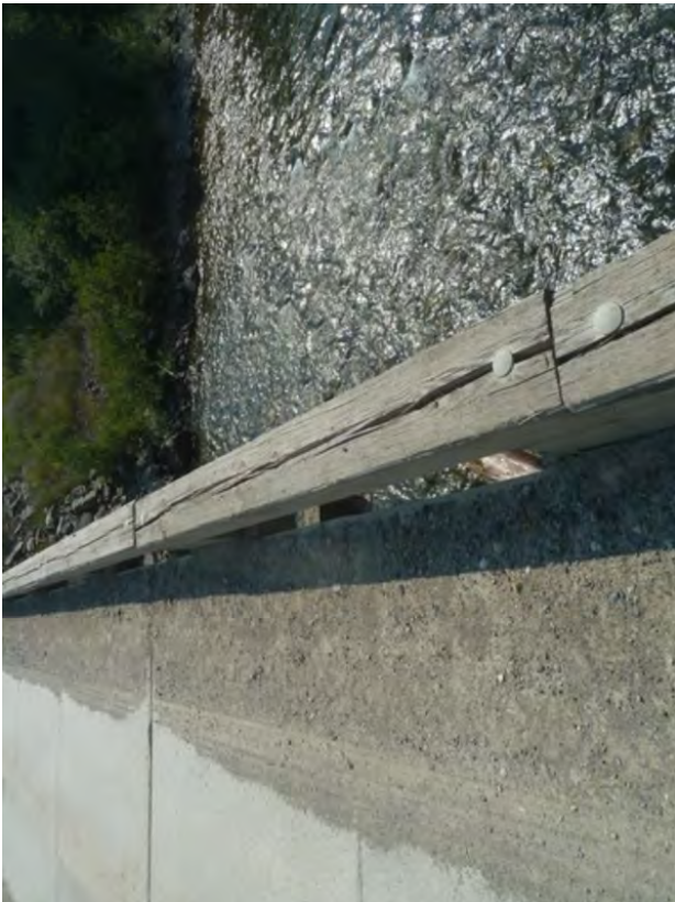
Figure 13: Wide checking in upstream curb.
