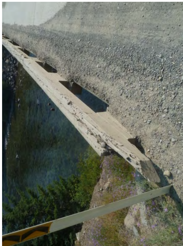
Figure 12: Damaged curb at left end downstream corner.
