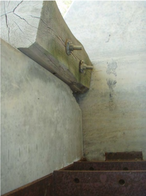
Figure 22: Deck panel at left end downstream - Note spalled concrete.
