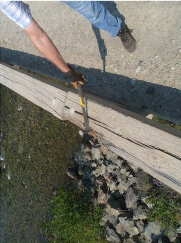
Figure 14: Rot in upstream curb near right end.
